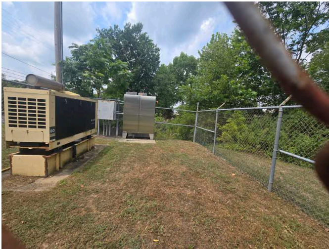
7. Pump B1 – Inside Fence
