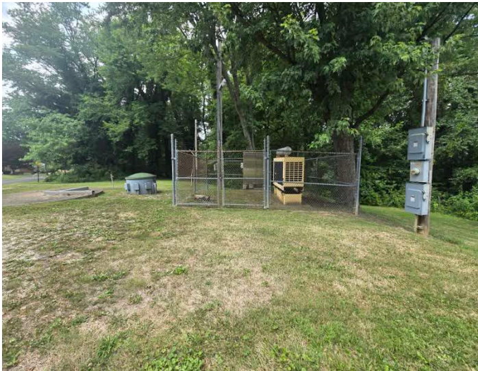
15. Pump Station B6 – Facing West – Close Up
