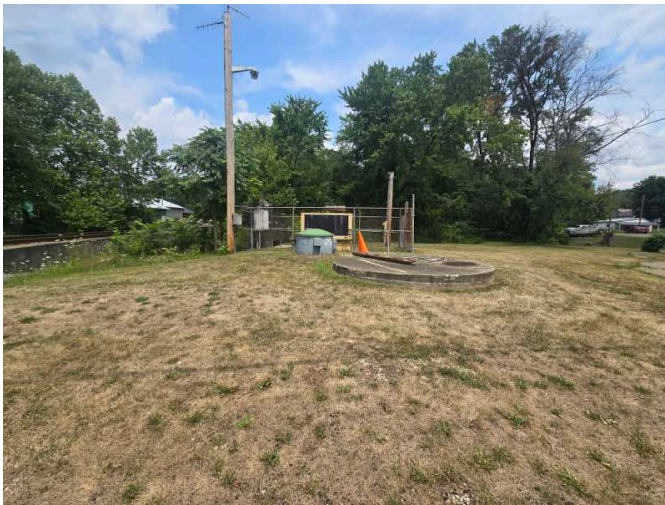
3. Pump B1 – Facing North
