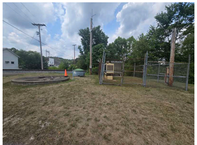
6. Pump B1 – Facing West – Close Up
