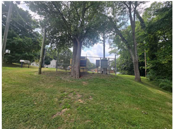
10. Pump Station B6 – Facing South
