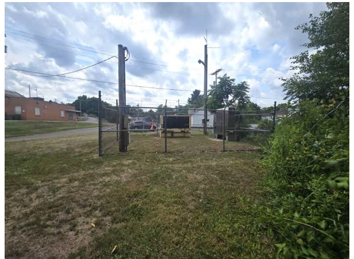
4. Pump B1 – Facing South
