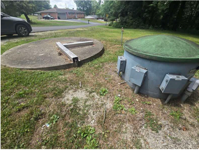
17. Pump Station B6 – Inside the fence.
