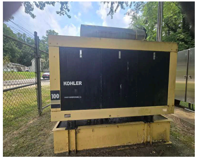
16. Pump Station B6 – Inside Fence
