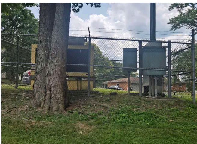
11. Pump Station B6 – Facing South Close Up
