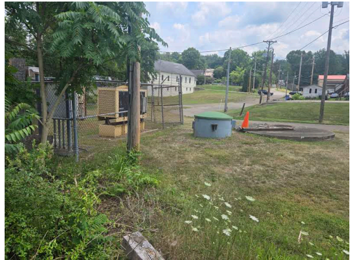
2. Pump B1 - Facing East – Close Up
