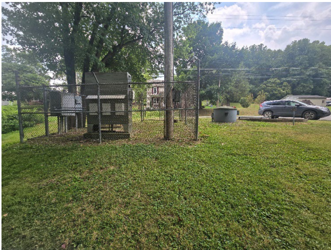
9. Pump B6 – Facing East – Close up
